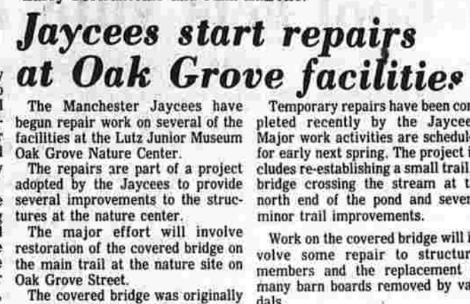
Manchester Jaycees make repairs to a foot bridge crossing a stream on a trail at the Oak Grove Nature Center. From left are Charles Rhoad, Randy Dumas, external vice-president, Larry Pietrantoni and John Labele.
